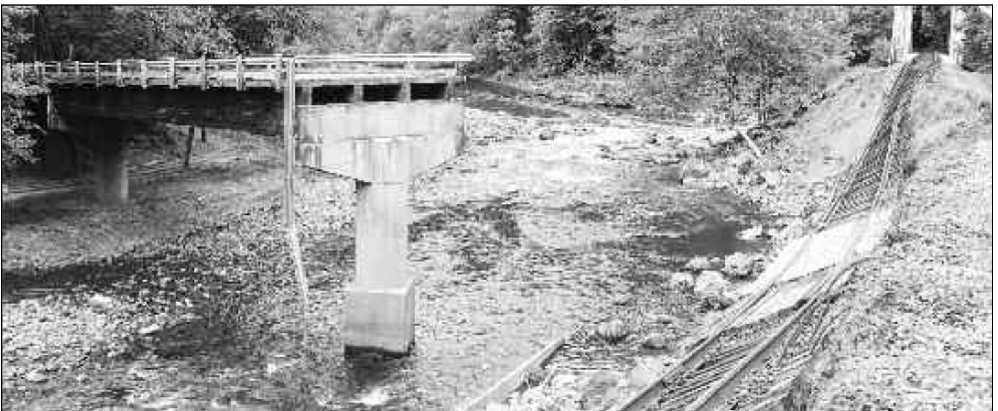
This county bridge across the Salmonberry river and the Port of Tillamook Bay Railroad were destroyed by the December 2007 flood. The bridge has been rebuilt, but the railroad wasn't able to come up with their 25% share of the estimated $57 million to repair flood damage. The railbed narrowed the canyon, exacerbating the fury of the flood.
